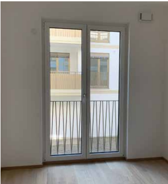
95% of all windows were floor-to-ceiling elements that were equipped with VSG according to the standard. MACO's Multi Mammut hardware was used for the high weights, says Matthias Buchegger, Project Manager at Heuberger Fenster (Fensterbau Salzburg).
